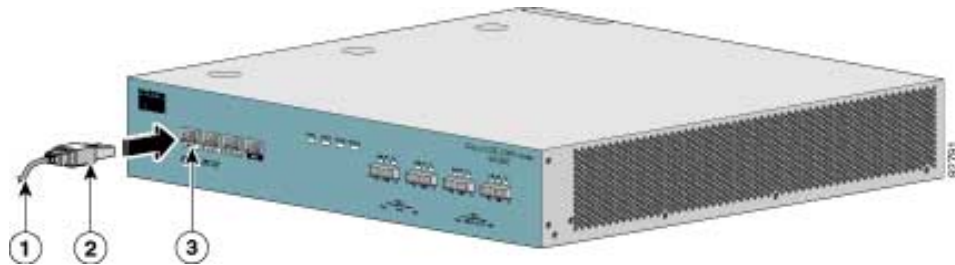
Figure 5-2: Cabling the Management Port
